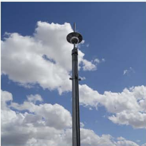
Lightning Protection and Grounding
